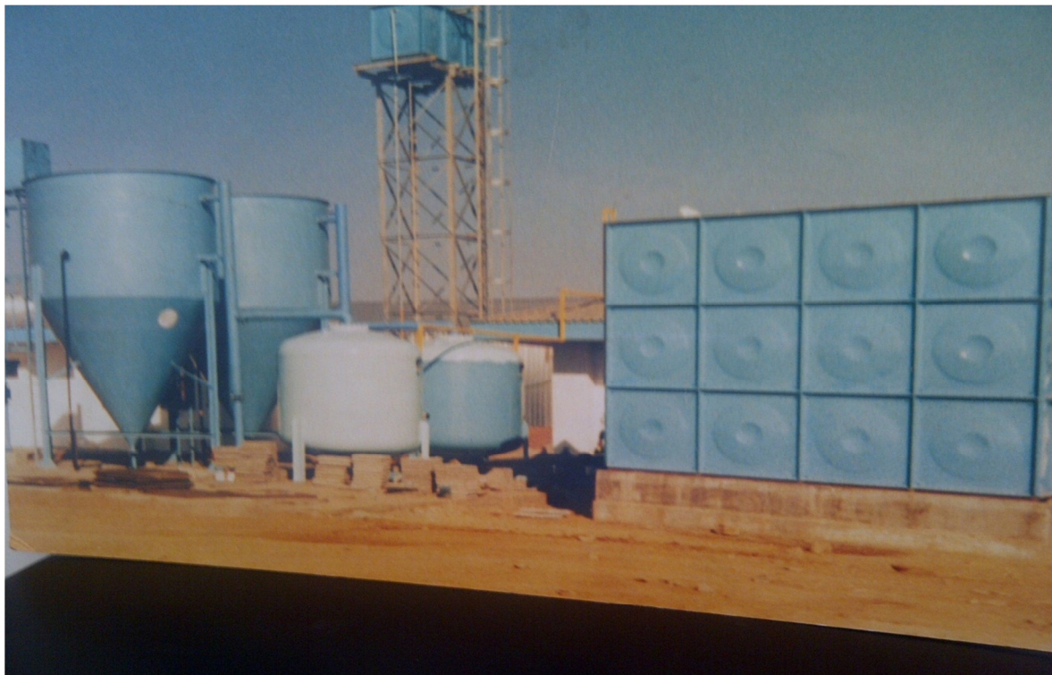
Typical plant installation showing Clarifiers, pressure type Sand Filters and Treated water storage tank.
