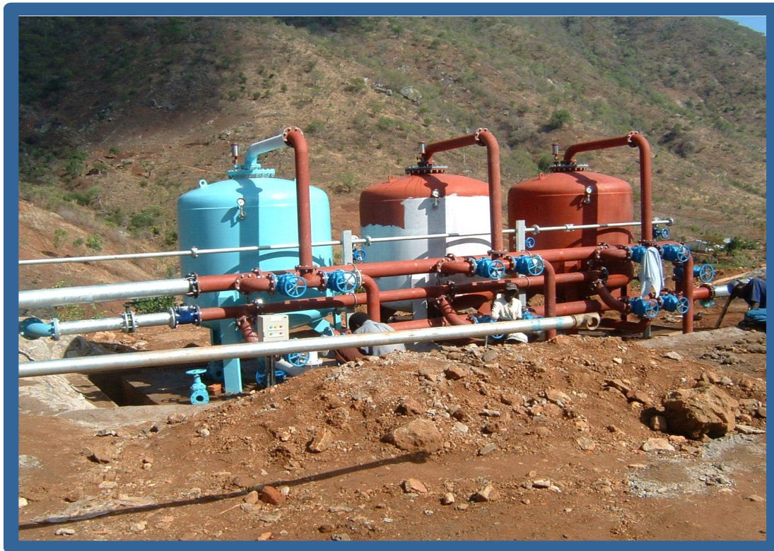
Installation of pressure type Sand Filters in a bank of three vessels.
